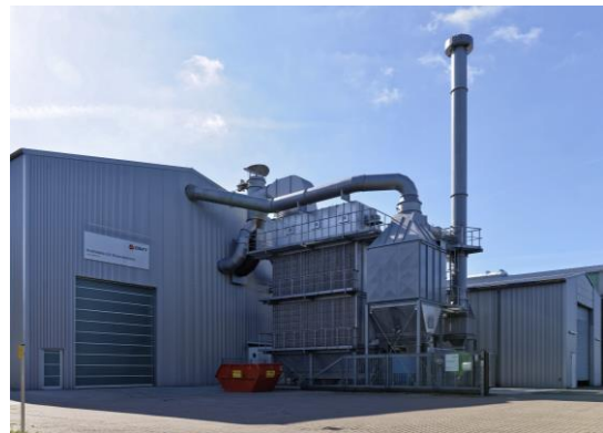
New test hall with flue gas cleaning system
